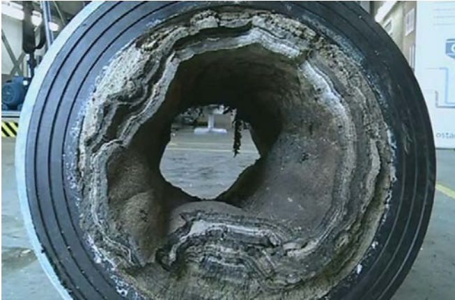
Ostara's nutrient recovery process will avoid problem deposits in pipes and valves
