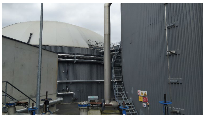
Cooperl site visit: anaerobic digesters
